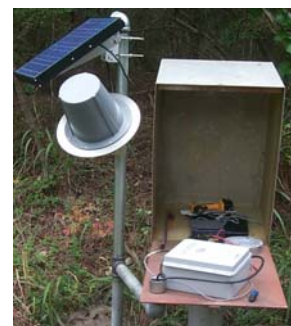
Figure 1 — Monitoring well with satellite telemetry equipment.
